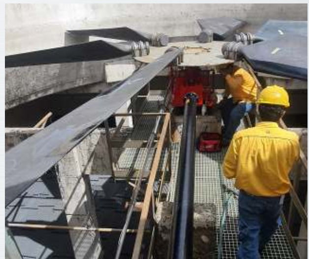
Local technicians during the installation of the MGS gearbox in one of the cooling towers.
